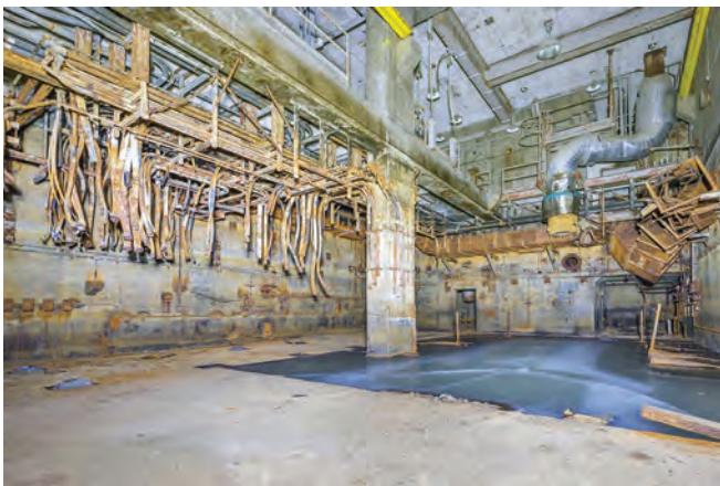
Contemporary photo of prime mover module 4. The generator bed is clearly visible under the ice. The combustion air room is through the doorway at the far end of the shot. The inaccessible mezzanine level is also visible. Photo Chris Howells
